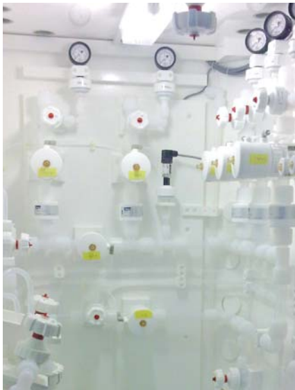
Chemical supply for wet processes
