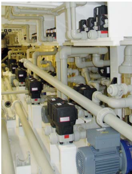
Media area of an etching and cleaning installation
