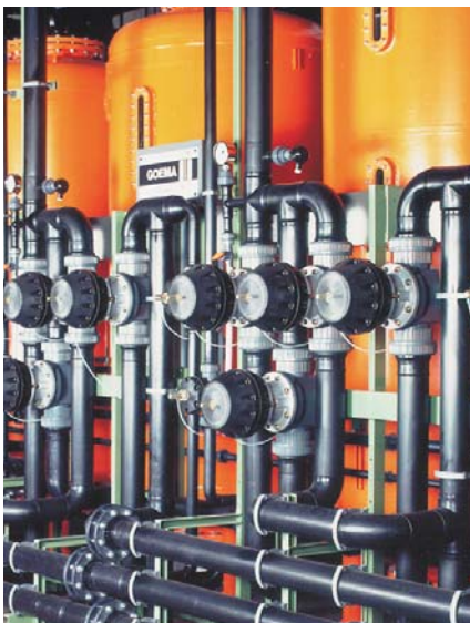
Waste water plant with PVC/PE components
