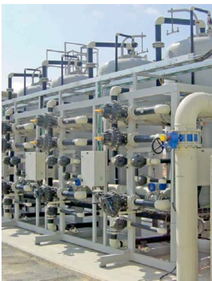
Water treatment (company Treitel Chemical Engineering LTD)
