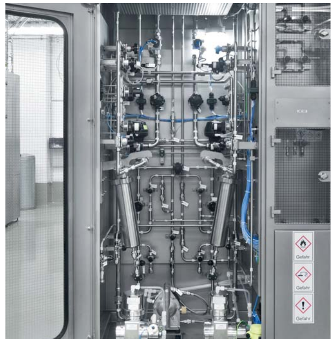
Detail of a solvent supply system (company Fäth)
