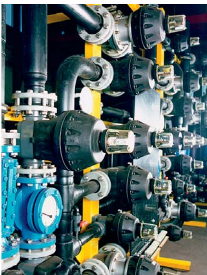
Waste water plant with PVC/PE components
