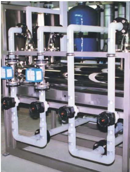
DI water treatment
