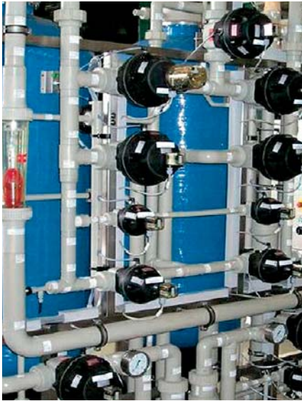
Plant with PP components
