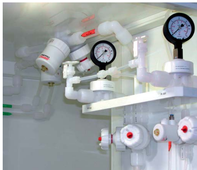
Detail of a chemical supply system
