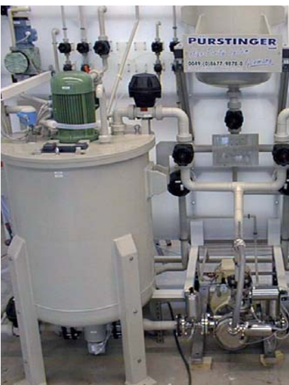
Slurry supply (company Puerstinger)
