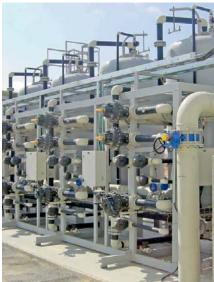
Water treatment (company Treitel Chemical Engineering LTD)
