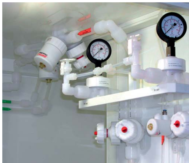
Detail of a chemical supply system
