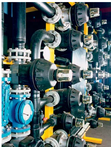
Waste water plant with PVC/PE components
