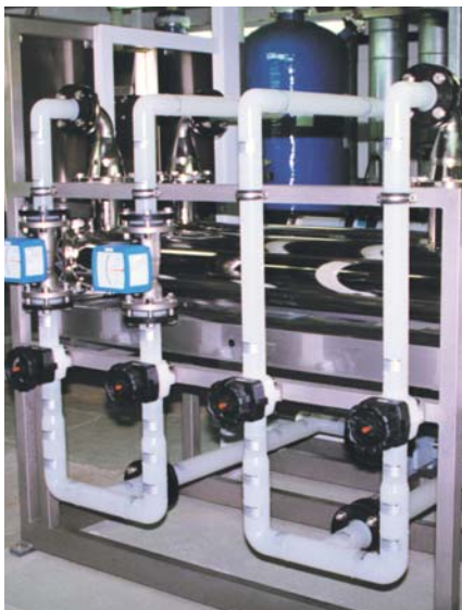
DI water treatment
